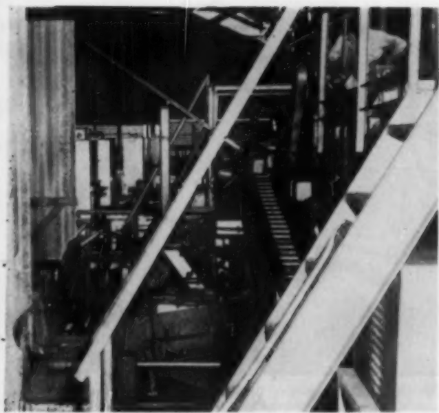
Billets move down the conveyor (upper right) to a transfer that assigns them to one of two forge furnaces. Limit switches at the furnace "tell" the transfer when a billet is needed. Billets roll down incline (center) and are sent to either of two lines through the furnace
